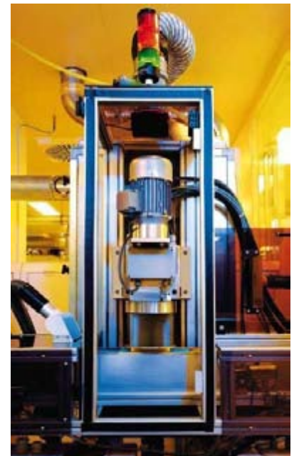
Photo Plasmatrete Fig.4. The circuit boards undergo a continuous process from the equipment via the plasma system through to the screen printing plant. Novotechnik's space-saving plasma plant serves four screen printing lines.
